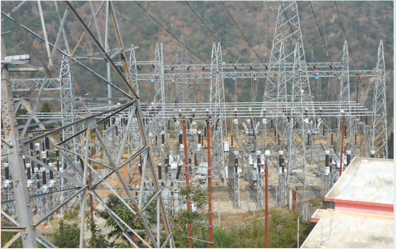
Receiving end of switchyard at Thapatar
