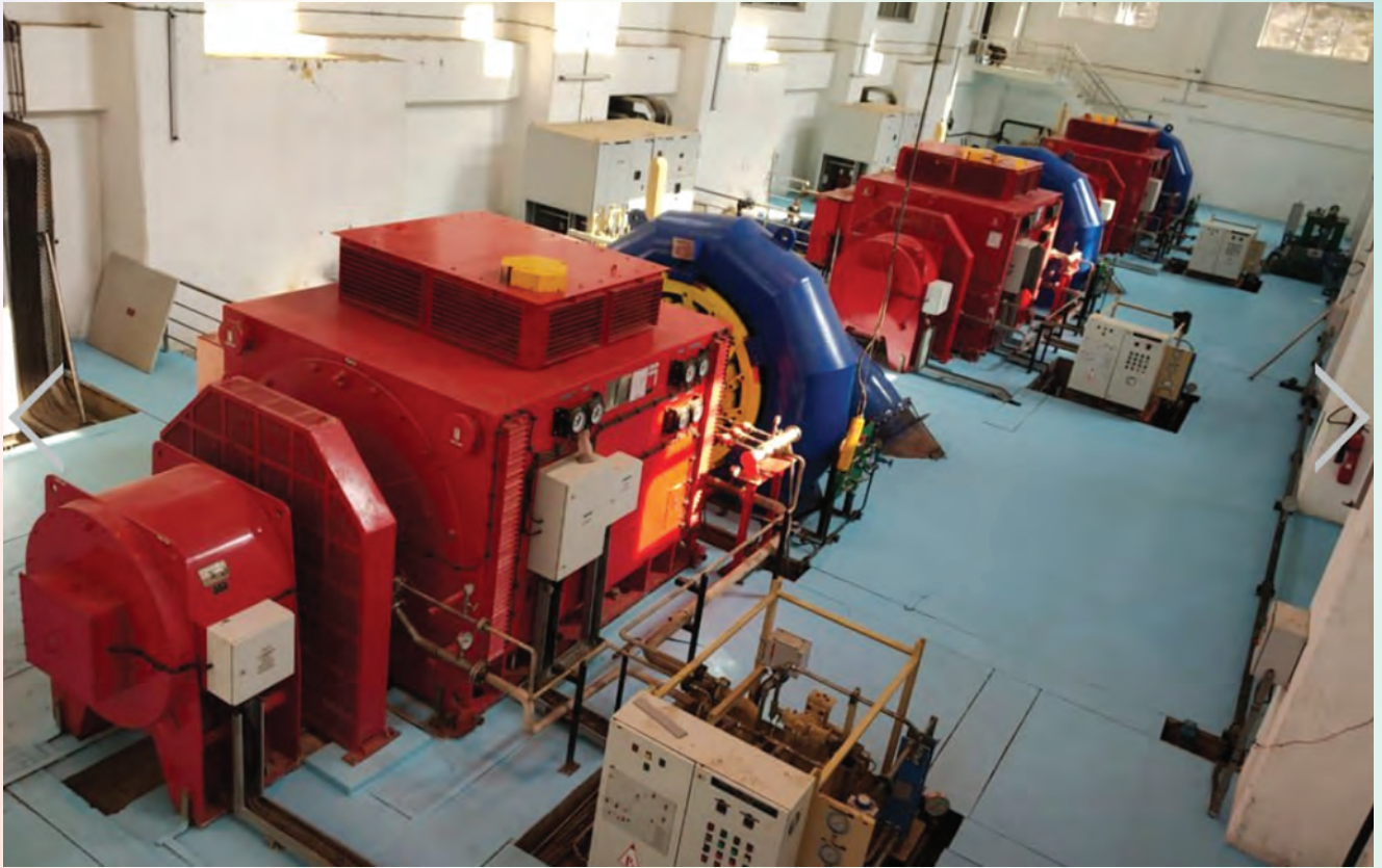
Turbine-Generator (Power House)
