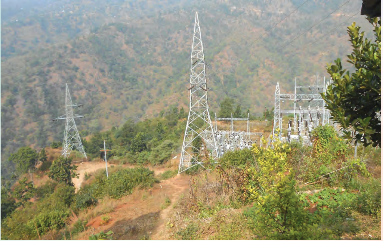
132 KVA Transmission Line (Tower no. 10 & 1)
