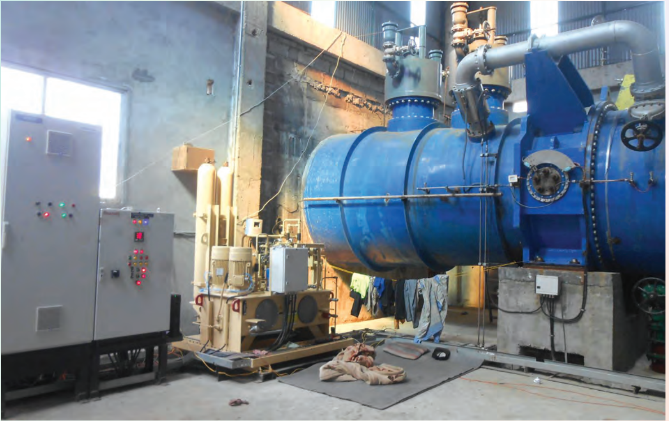
Penstock protection valve
