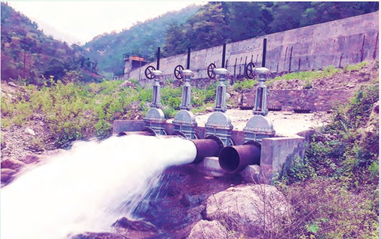
Hewa sand flushing
