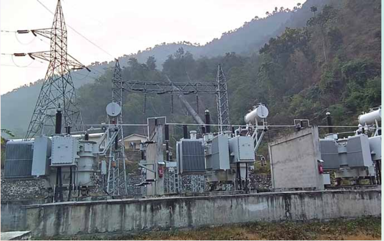
Sending end of switchyard at Powerhouse
