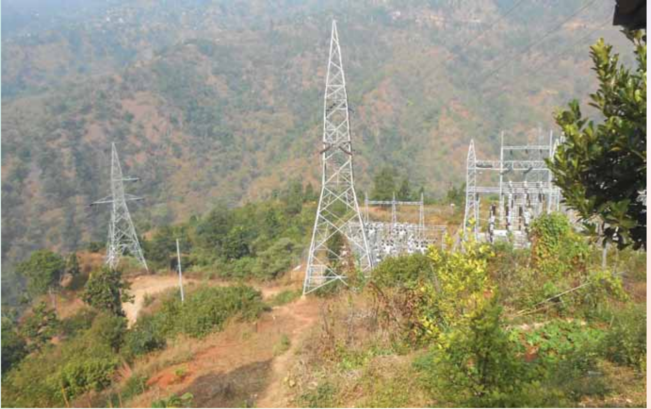
132 KVA Transmission Line (Tower no. 10 & 11)
