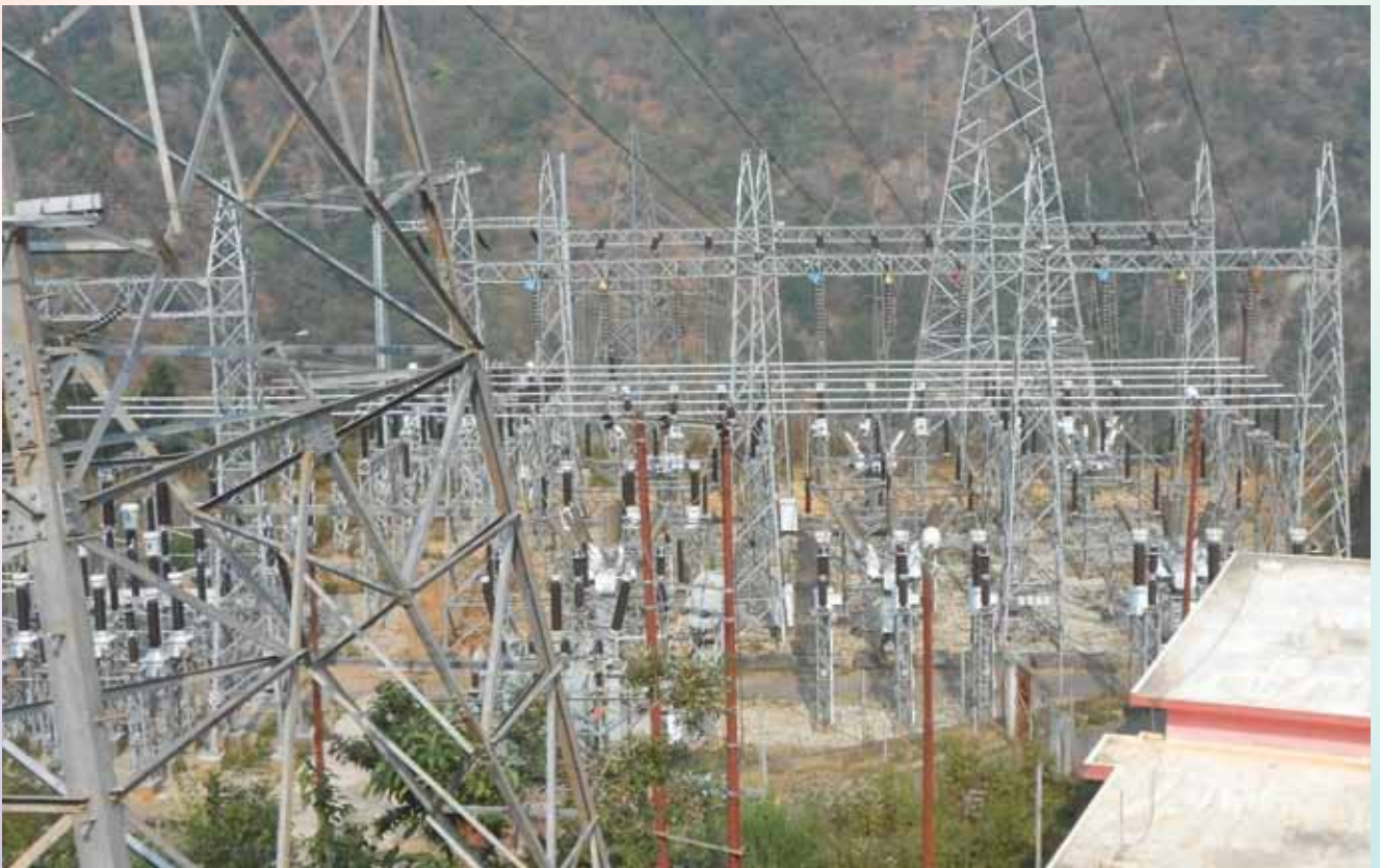
Receiving end of switchyard at Thapatar
