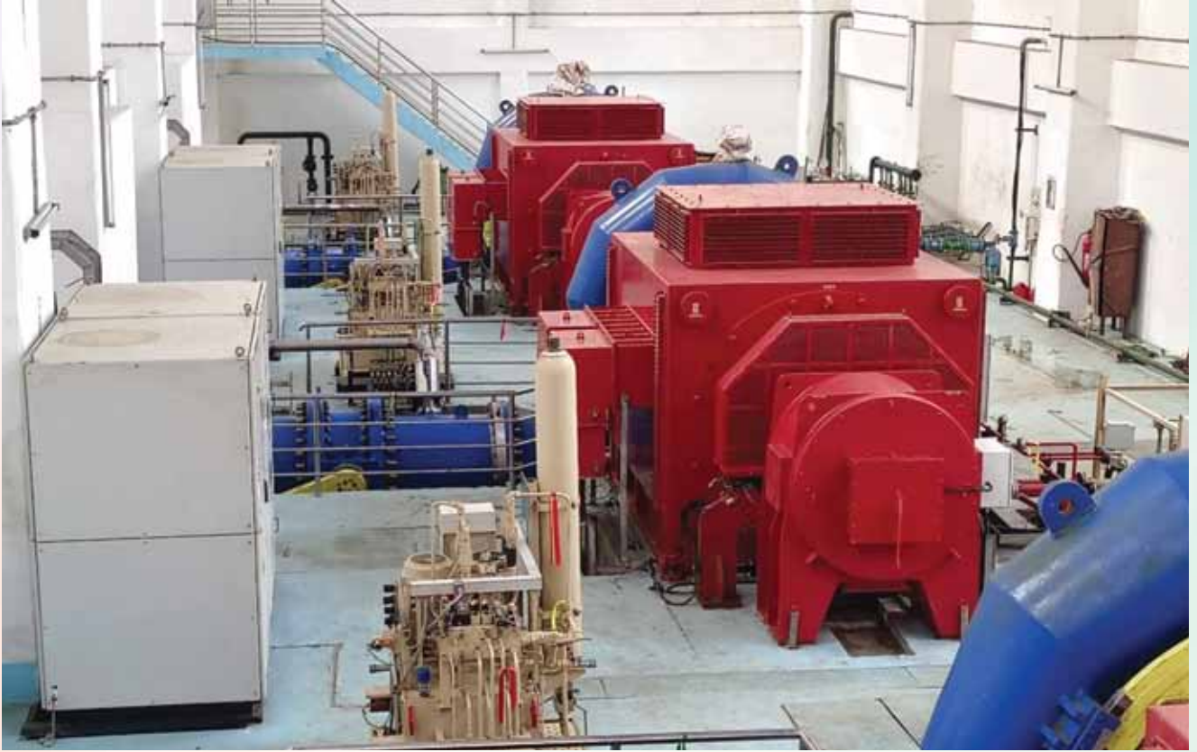
Turbine-Generator (Power House)
