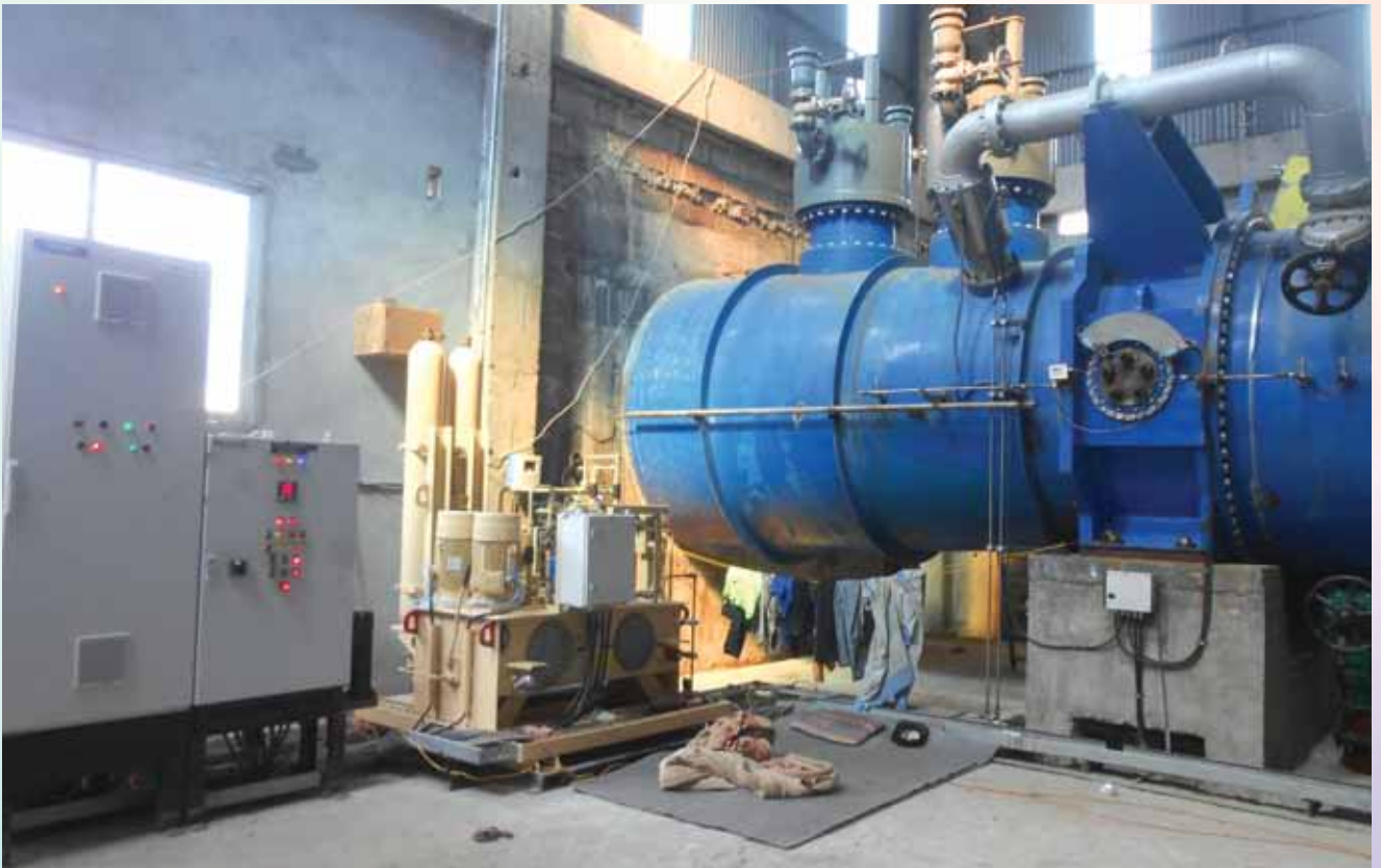
Penstock protective valve
