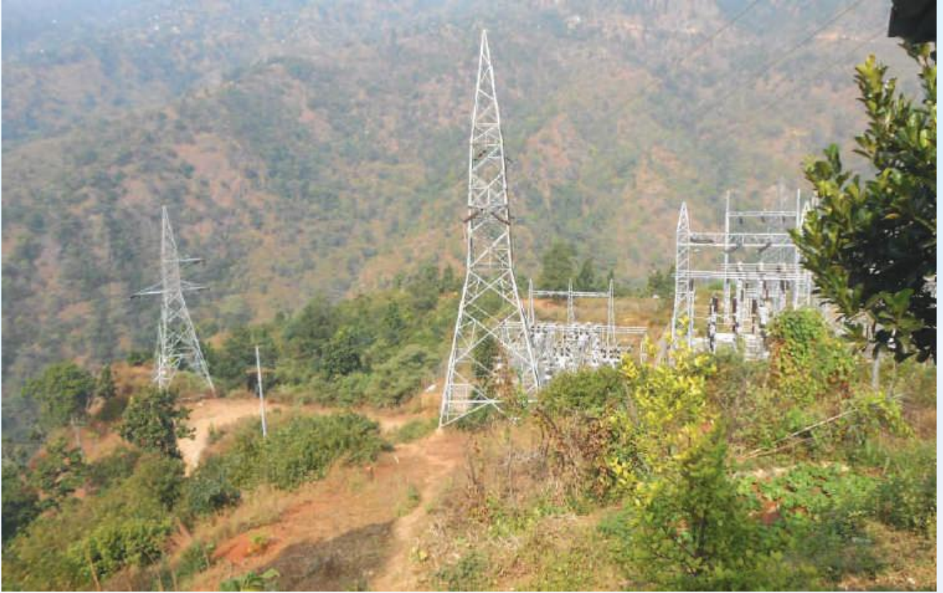
132 KVA Transmission Line (Tower no. 10 & 1)
