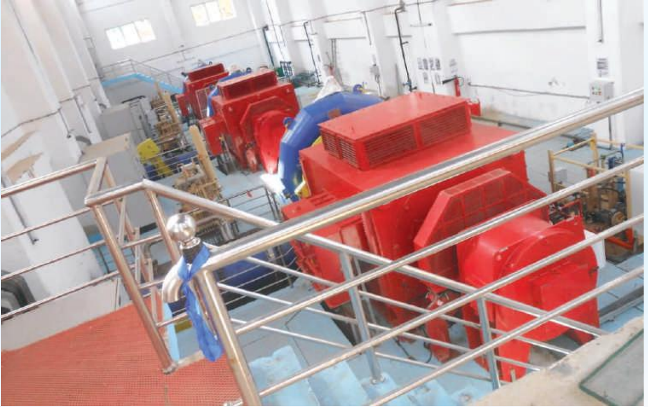
Turbine-Generator (Power House)
