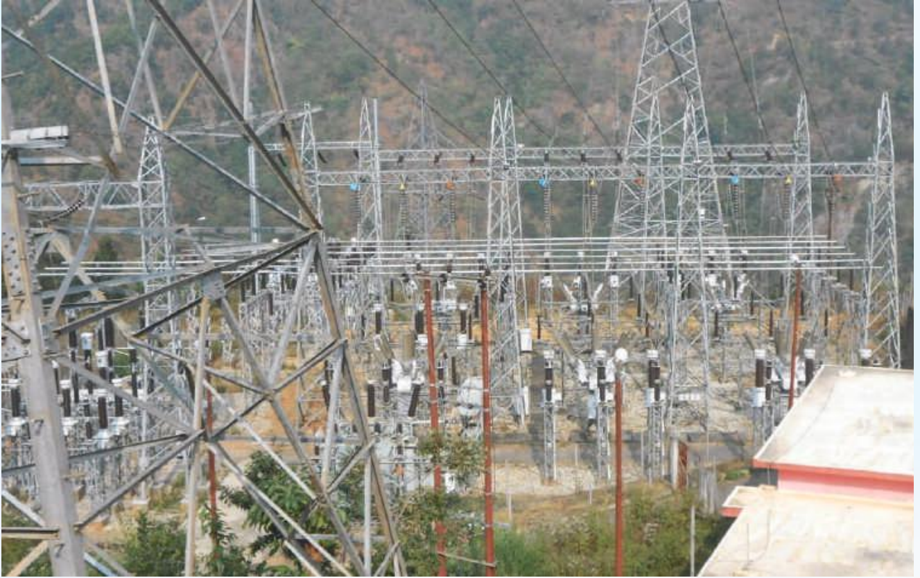
Receiving end of switchyard at Thapatar
