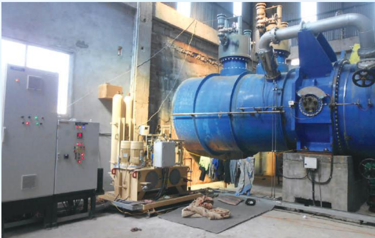
Penstock protection valve
